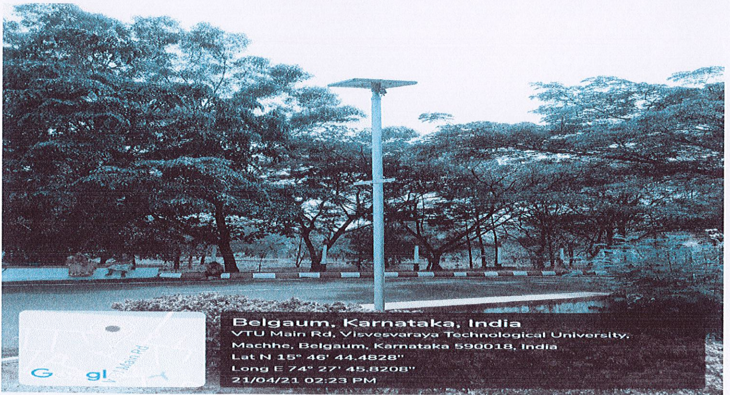
Solar panel at VTU Main road
