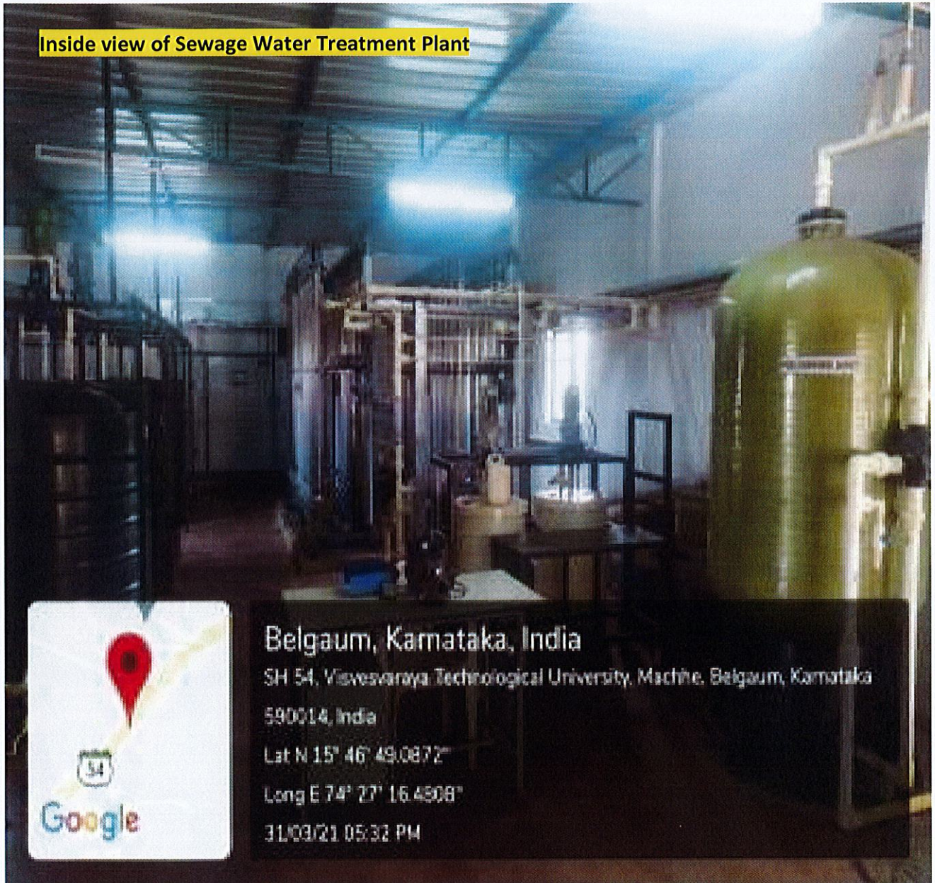
Sewage Treatment Plant
